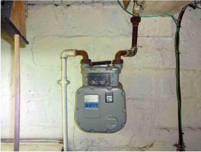
Fuel / Gas Service - BASEMENT
