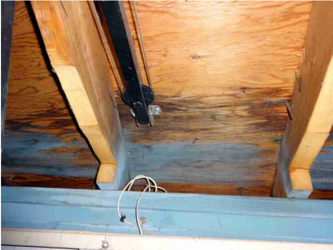
Roof Covering - OTHER LIFTED SHINGLE NOTED WHICH APPEARS TO BE BECAUSE OF THE GARAGE DOOR OPENER RAIL MOUNTING
