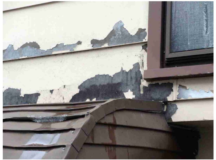
Siding - MINOR DECAY / DAMAGE / PEELING / CRACKING / CORROSION - These areas should be scraped, primed, and painted or stained. Any decayed / damaged sections should be replaced.
