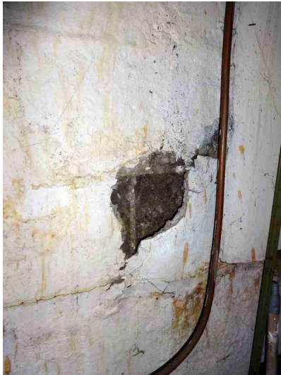
Type / Location / How accessed / Viewed / Condition - Spalling Noted - INTERNAL Spalling is the deterioration of the masonry surface. This takes place due to moisture behind the wall. The source of moisture should be located and eliminated.
