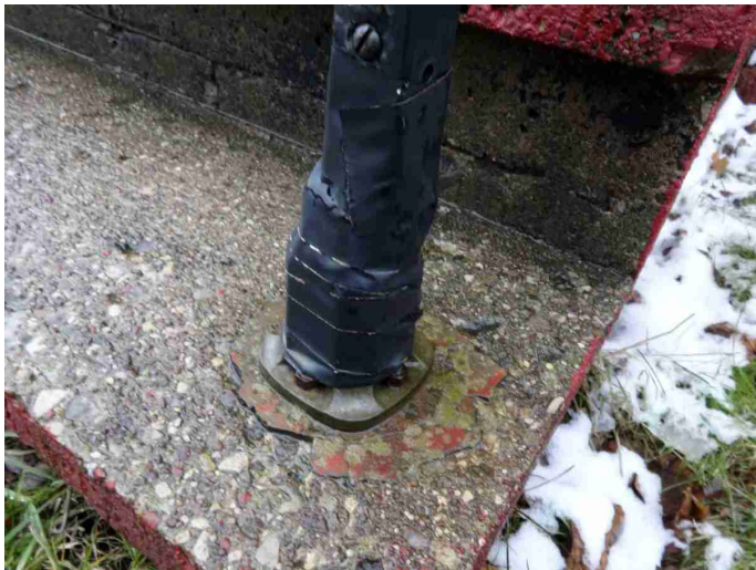
Deck / Porch / Patio / Balcony - INSTALL / REINFORCE / REPLACE HANDRAILINGS The railings should be replaced or rebuilt for safety. ELECTRICAL TAPE NOTED AT THE FRONT PORCH RAILING
