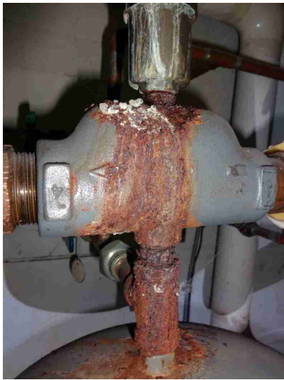
Location / Type / Distribution - OTHER CONSIDERABLE CORROSION NOTED AT THE BACK-FLOW PREVENTER / EXPANSION TANK
