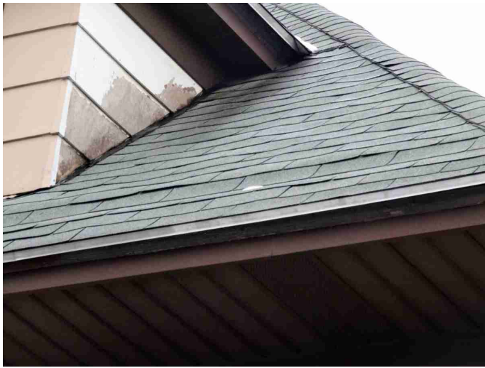
Siding - MINOR DECAY / DAMAGE / PEELING / CRACKING / CORROSION - These areas should be scraped, primed, and painted or stained. Any decayed / damaged sections should be replaced.
