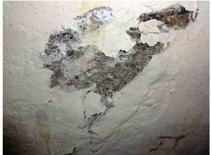
Type / Location / How accessed / Viewed / Condition - Spalling Noted - INTERNAL Spalling is the deterioration of the masonry surface. This takes place due to moisture behind the wall. The source of moisture should be located and eliminated.
