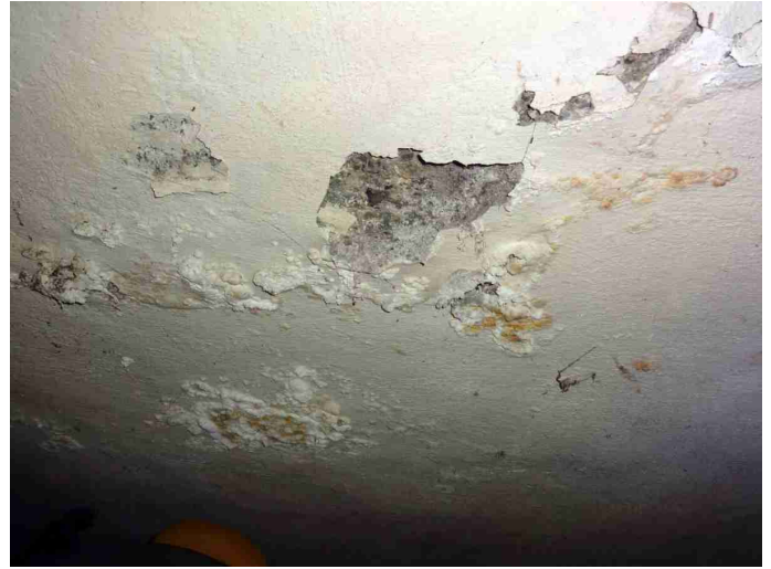
Type / Location / How accessed / Viewed / Condition - Spalling Noted - INTERNAL Spalling is the deterioration of the masonry surface. This takes place due to moisture behind the wall. The source of moisture should be located and eliminated.
