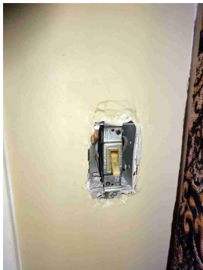
Wiring (Branch Circuit) - DAMAGED / MISSING OUTLET / SWITCH COVERS The covers should be replaced for safety reasons. Exposed receptacles / switches could lead to electric shock.
