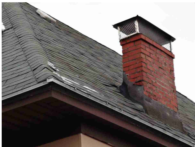
Roof Structure - (viewed from Exterior) - SLIGHT IRREGULARITIES NOTED
