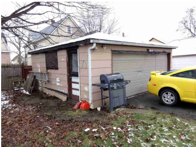
Garage Type / Materials / General condition - MINOR DECAY / DAMAGE
